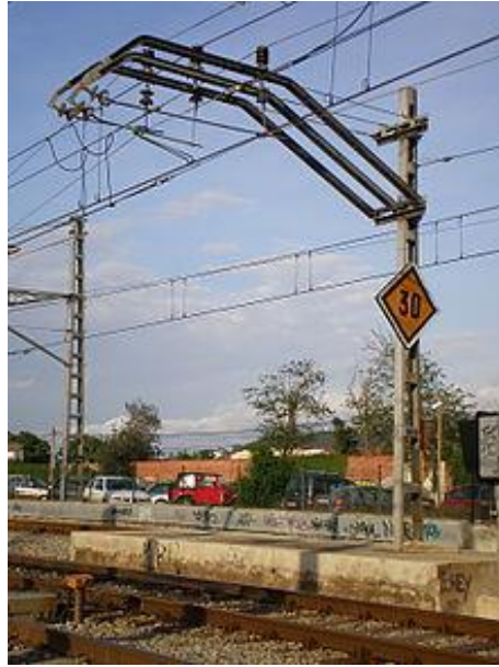
Figure 5. OCS temporary foundation
