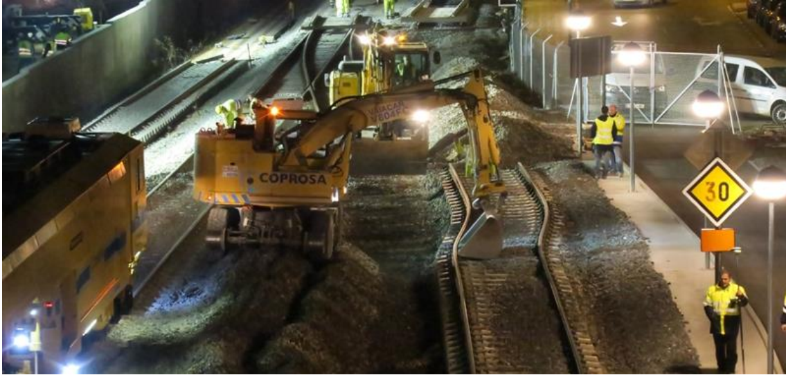
Figure 4. Lateral Displacements of the track greater than 21.34 ft
