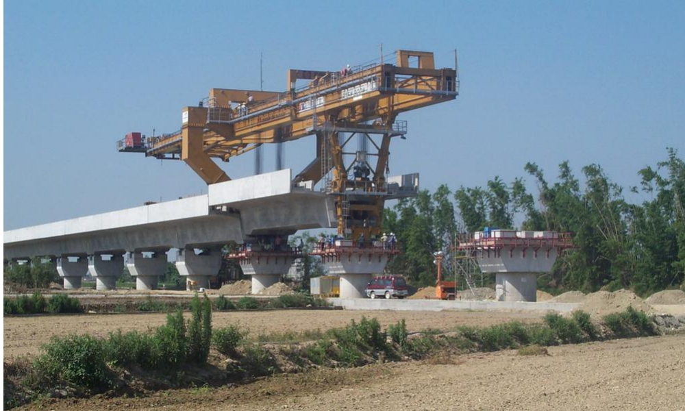
Figure 6-4: Example of Overhead Gantry
