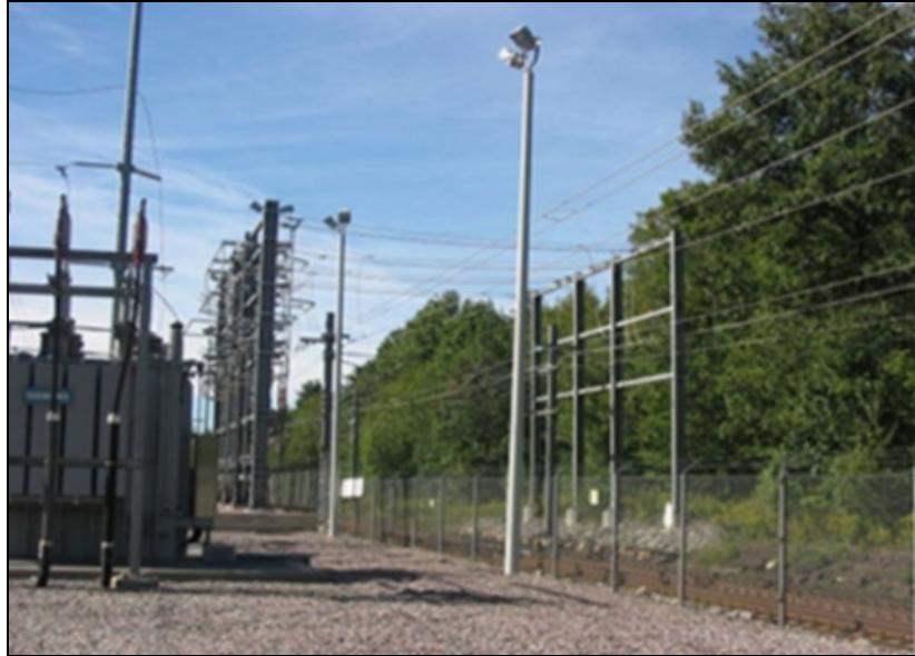
Figure 2-28 Paralleling Station Overhead Contact System Gantry
