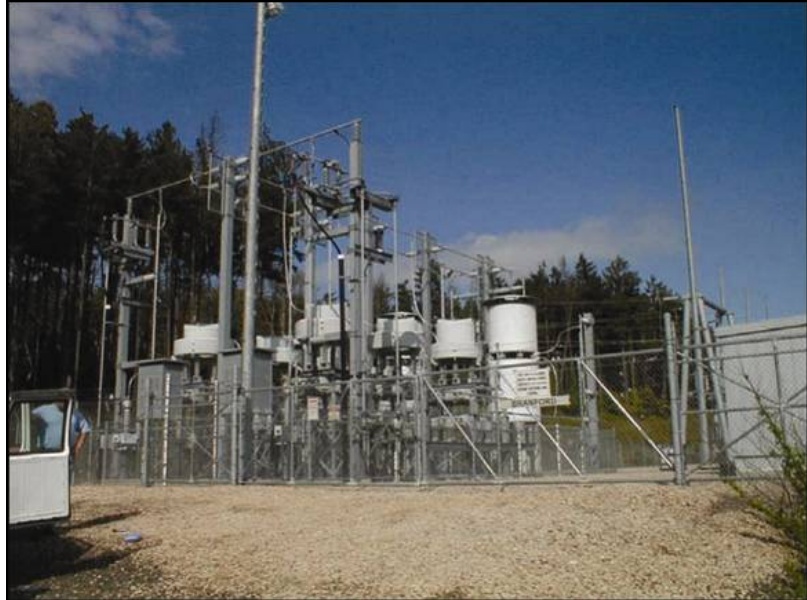
Figure 2-24 Traction Power Substation
