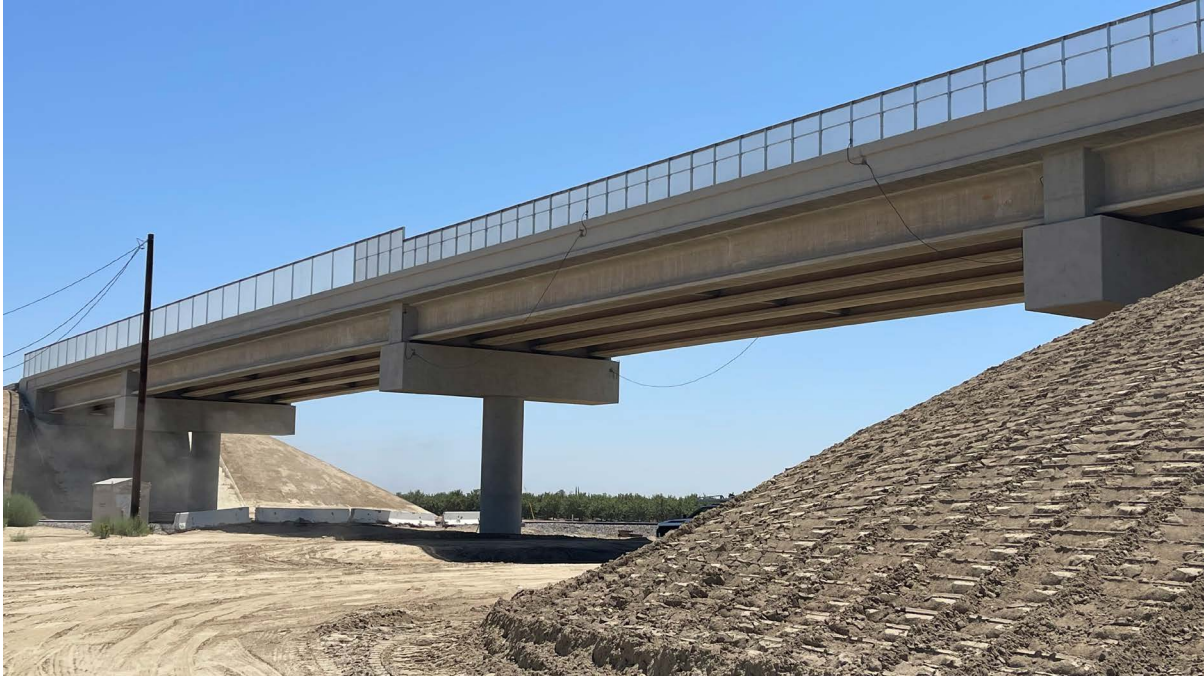
Fencing can be seen atop the Floral Avenue Grade Separation in Fresno County. The structure opened to traffic on July 15, 2024
