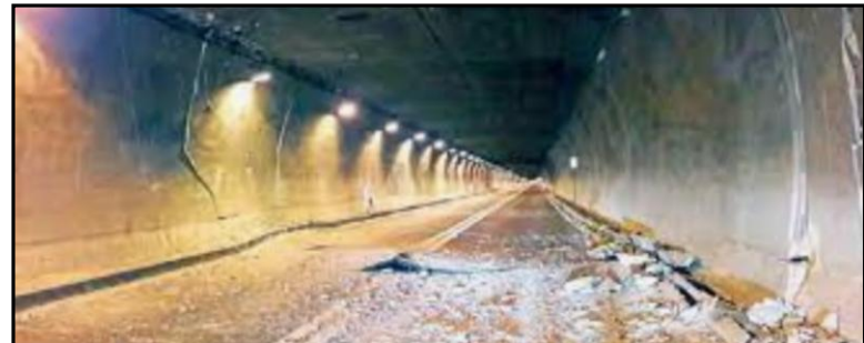
2016 San Benedetto tunnel following the Norcia earthquake in Italy.
