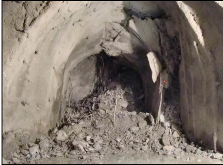
Rock burst in a Chinese tunnel
