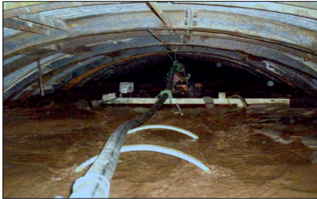
Photo: Parbati TBM buried in silt
