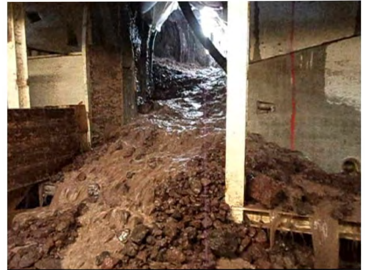
Photo Caption from the Robbins Company white paper on the Gerede Project: Of the three standard Double Shield TBMs used to originally bore sections of the tunnel, two became irretrievably stuck or damaged amid massive mud and water inflows.
