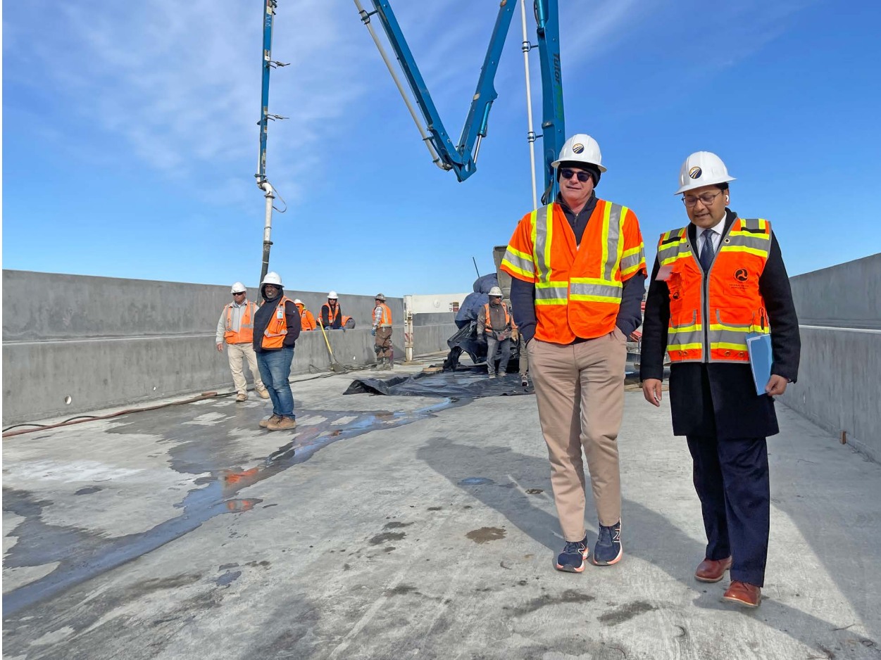
Photo: CEO Brian Kelly and FRA Administrator Amit Bose tour the Cedar Viaduct in Fresno
