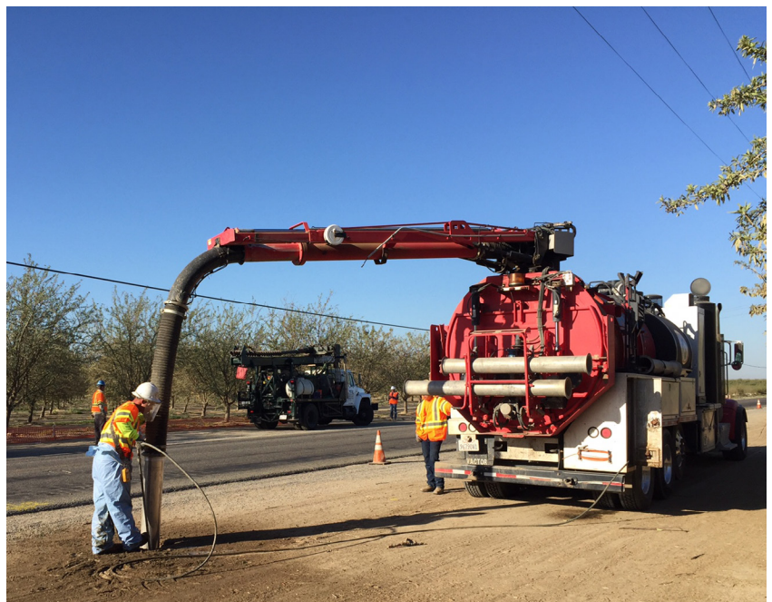
Pre-construction activities getting underway Construction Package 4 in October with “pot holing”. During this process crews locate utilities to in order to avoid them during construction. In some cases, utility relocation is necessary.
