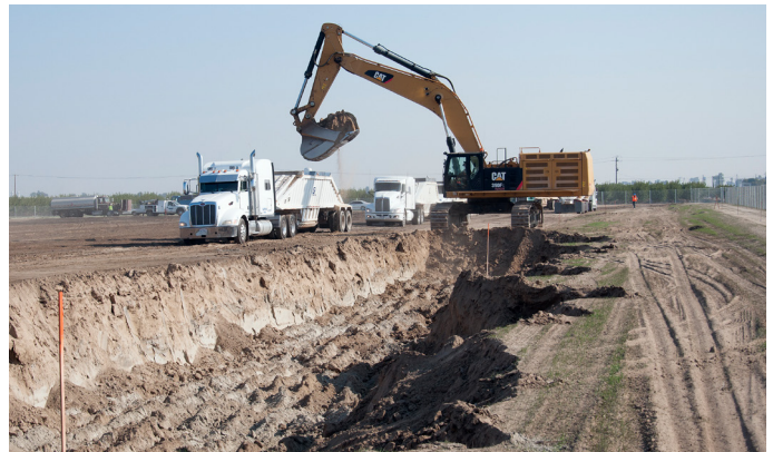
The first construction work in Construction Package 2-3 getting underway in November 2016 with the building of a test berm in Fresno County. Crews in CP 2-3 have also been busy with several road paving projects.
