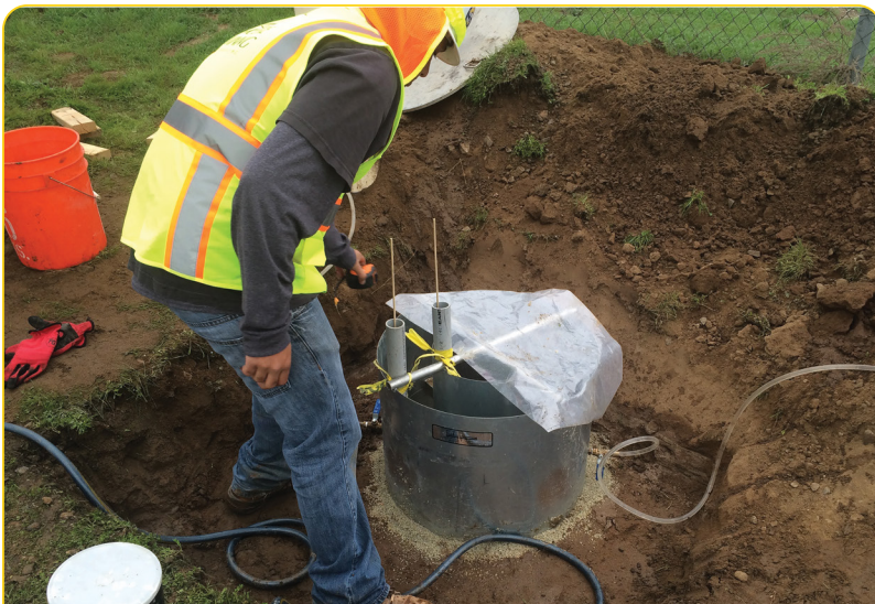
Disabled Veteran Business Enterprise Moore Twining conducted procedures known as infiltration testing as part of our permitting agreement with the State Water Quality Control Board. The testing included sensors which measured the rate at which water is absorbed into the ground as part of work on CP 1.
