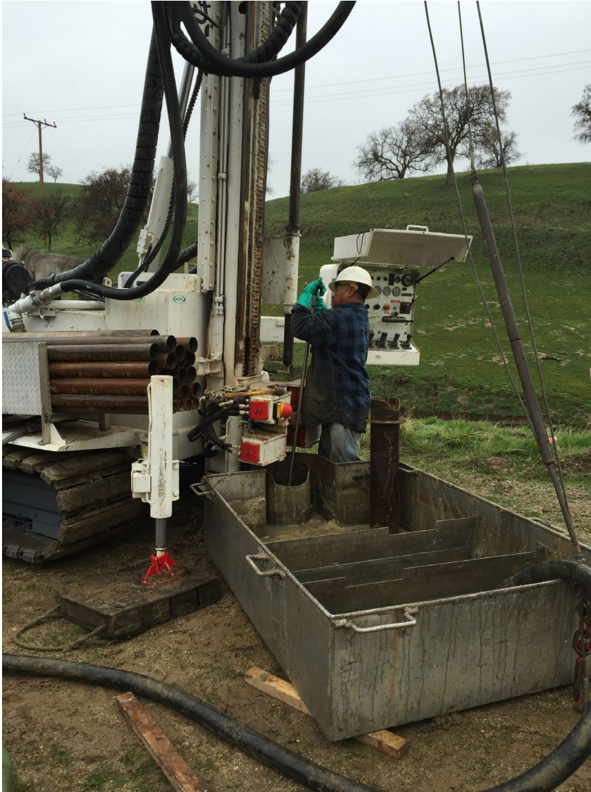
A member of EMI's drilling team setting up on a hole along the Bakersfield to Palmdale project section.
