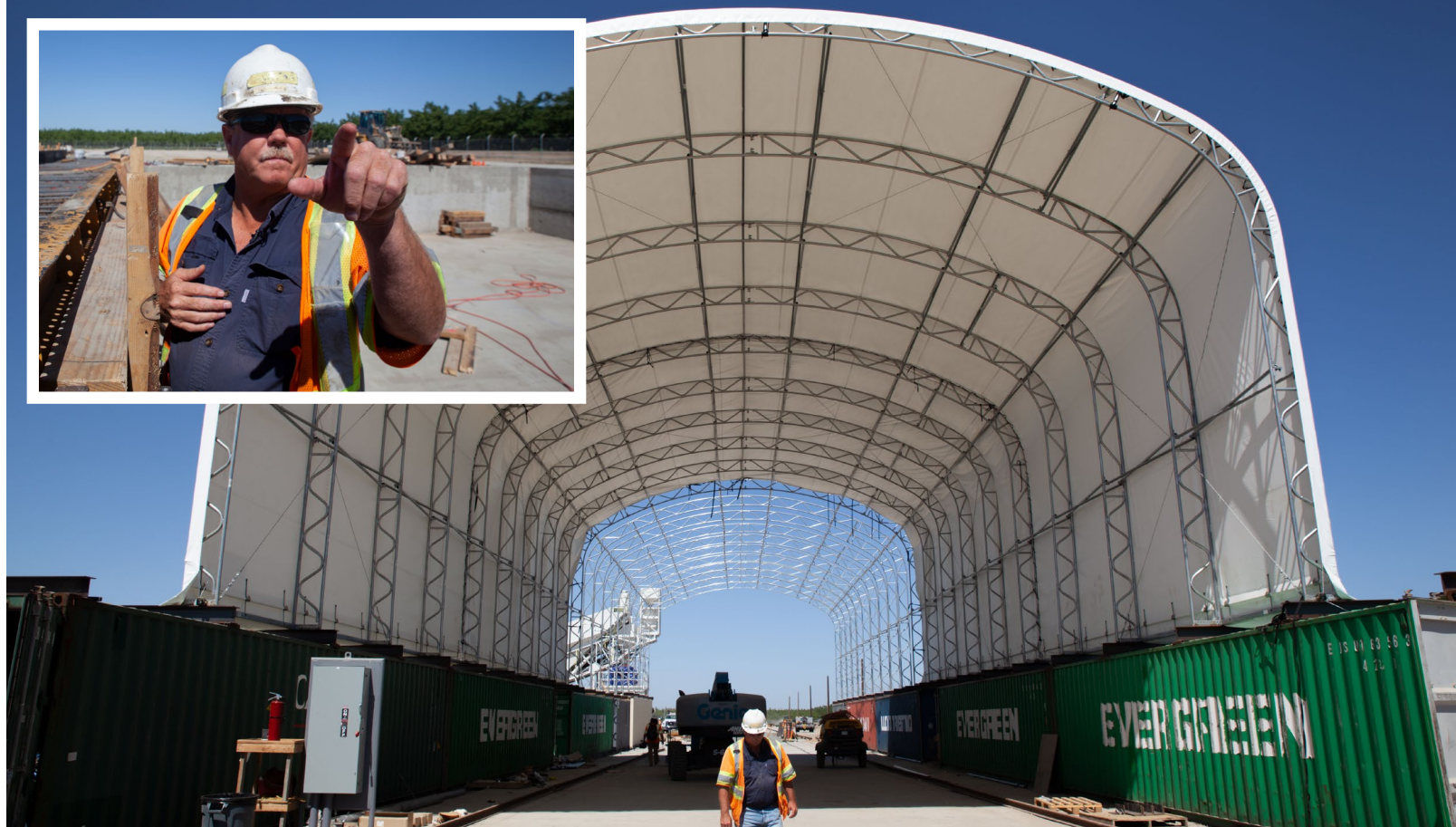
Design-builder Dragados Flatiron Joint Venture is building a precast facility outside Hanford to make girders for Construction Package 2-3. Mick Wilson (inset) is the project superintendent.
