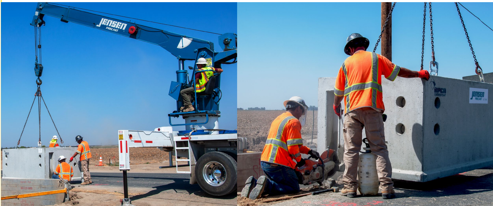
Thirteen employees for Leo Tidwell Excavating Corporation are dedicated to working on the high-speed rail project. They are moving underground utilities for AT&T. The firm has contracts to work on sites in Construction Package 2-3 and Construction Package 4, worth a total of about $9.5 million.
