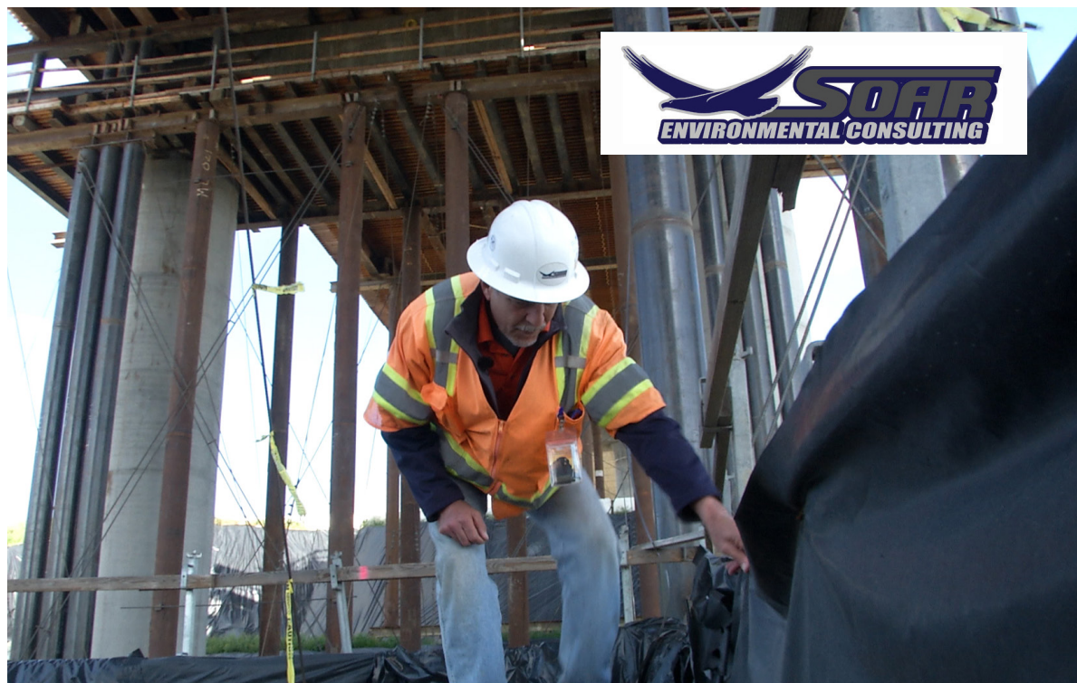
Evan Studley checks plastic sheeting at the San Joaquin River viaduct to ensure construction work isn’t allowing dirt or sediment to leak into the San Joaquin River and harm fish and other animals just north of Fresno. Every week, Studley walks the site located north of Fresno. Studley is a program manager for Soar Environmental Consulting. He also serves as Storm Water Pollution Prevention Plan oversight coordinator for the high-speed rail project.
