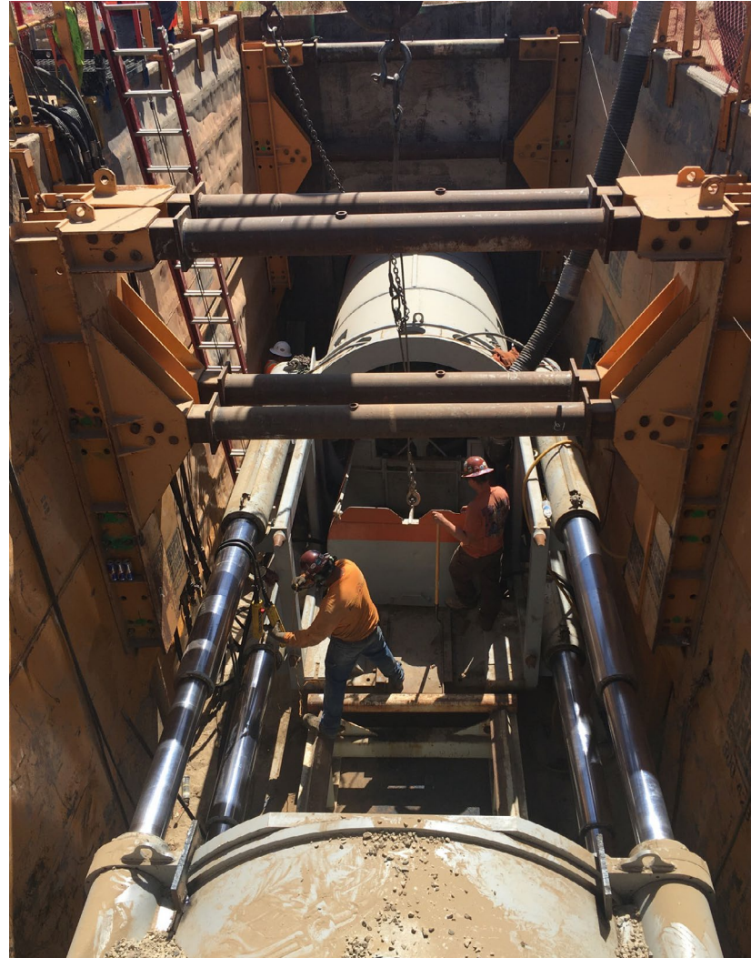
The high-speed rail project has more than a thousand utility relocations, which can range from PG&E poles, AT&T lines, to irrigation lines
