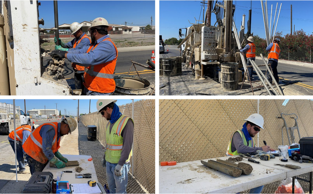
In June 2022, crews from Gregg conducted geotechnical drilling with mud rotary methods and Standard Penetration Testing (SPT) sampling. (Central Valley) Lead driller: Sam Gutierrez, Assistant driller: Martin Chavez
