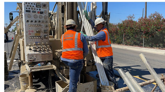
Tremie Pipe is used to grout up the completed boreholes created by Gregg Drilling crews in June 2022 working on the Shafter to Bakersfield stretch of the alignment in the Central Valley. Lead driller: Sam Gutierrez, Assistant driller: Martin Chavez
