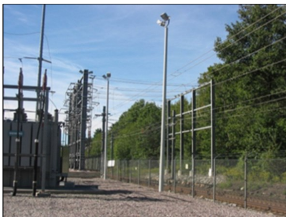
Figure 2-29 Paralleling Station Overhead Catenary System Gantry
