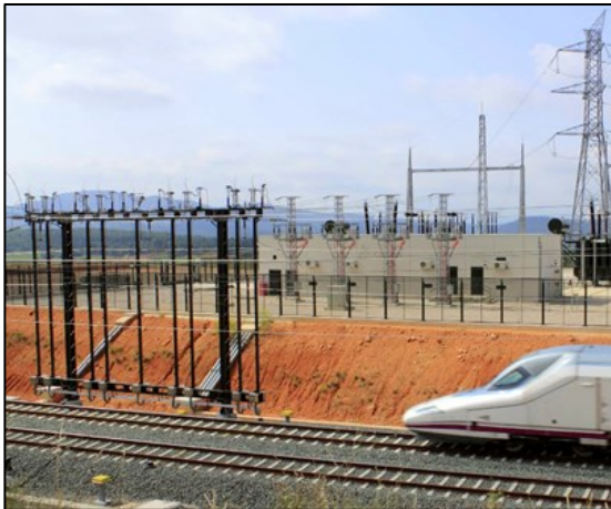
Figure 2-25 Traction Power Substation
