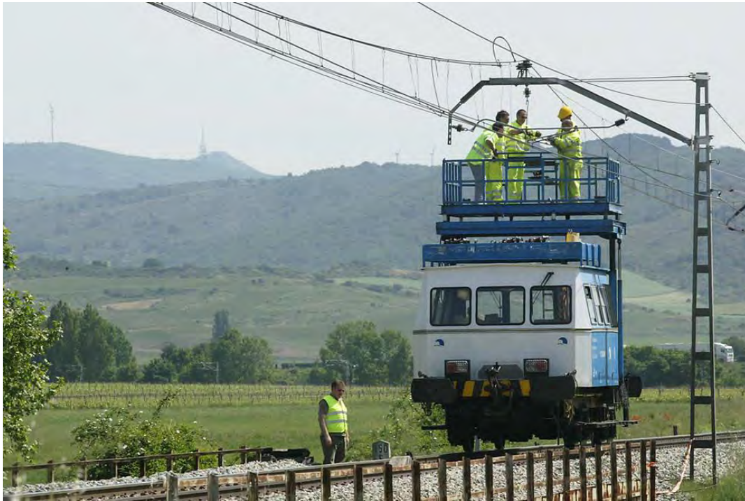
Figure 12. Horizontal and Vertical adjustment of contact wire
