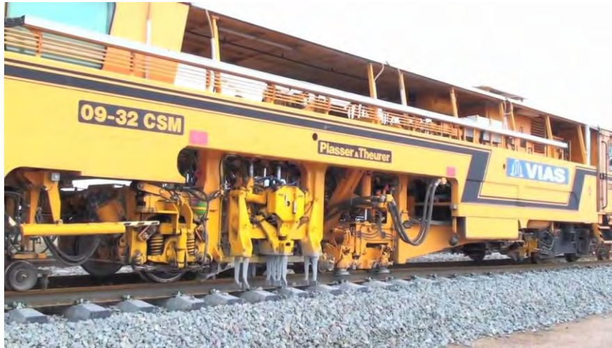
Figure 2. Tamping machine used for lateral displacements of the track between 0 and 1 ft.
