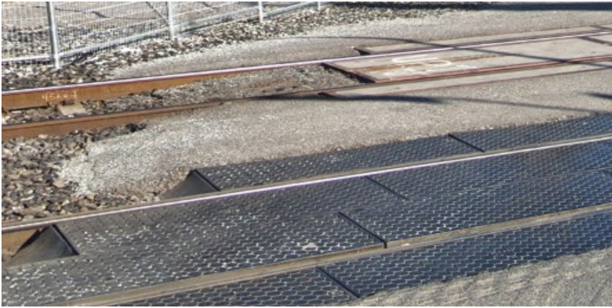
Figure 2. Platform for vehicular passage on the tracks.
