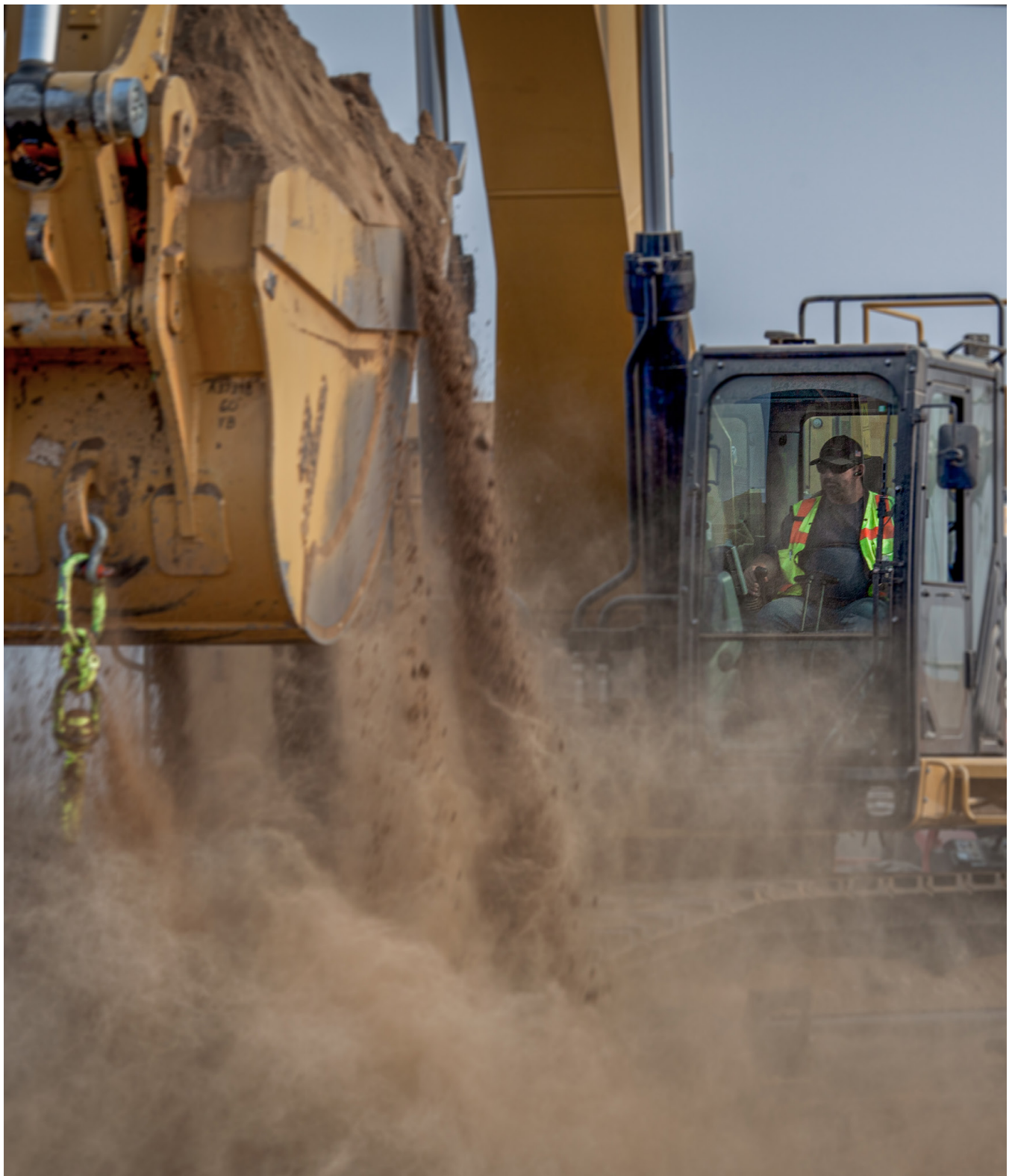
PHOTO: Work continues on Construction Package 2-3 at South Avenue in Fresno County.
