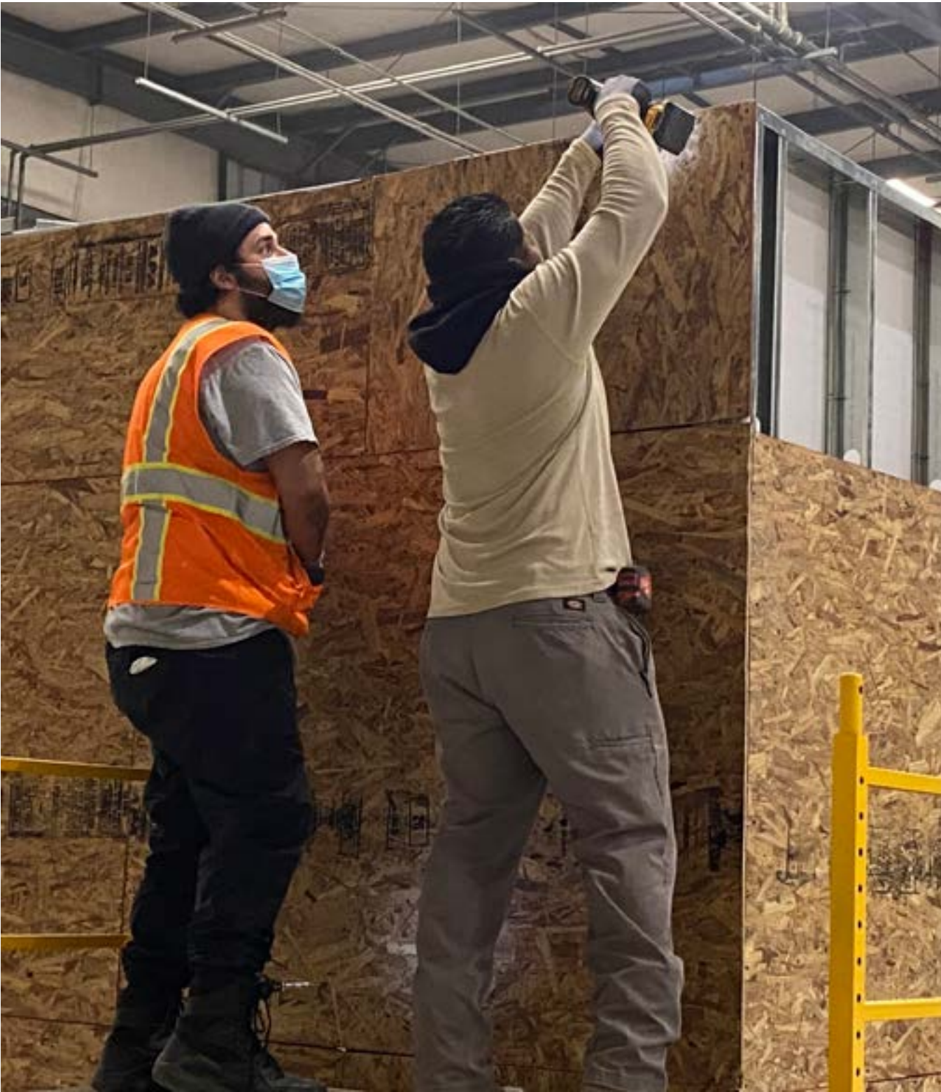
PHOTO: Students at the Central Valley Training Center learn important skills in the construction trades.
