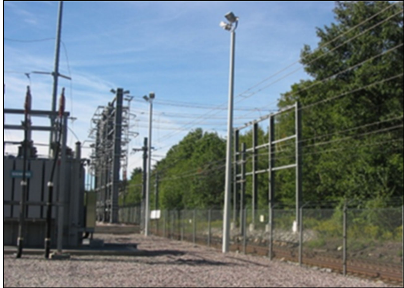
Figure 2-28 Paralleling Station Overhead Contact System Gantry
