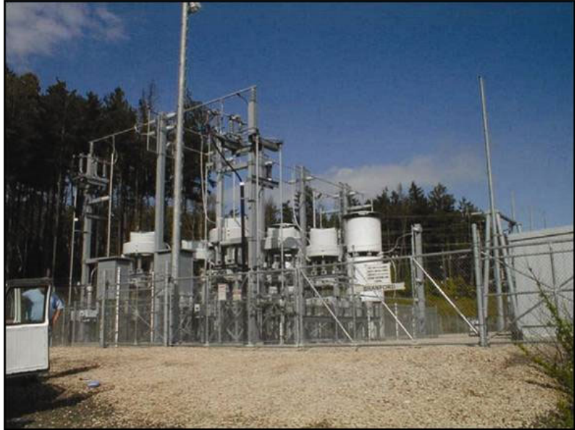
Figure 2-24 Traction Power Substation
