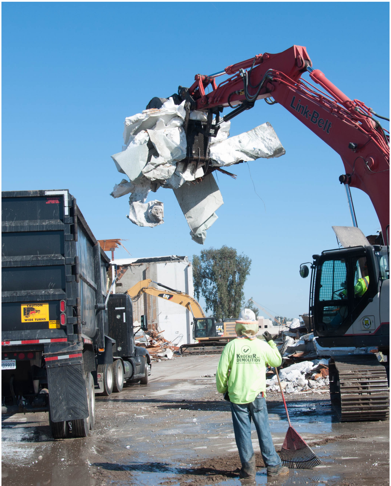
PHOTO: Since 2015, more than 272,000 tons of material, including concrete, asphalt, wood and organics, have been stockpiled for reuse or recycled as part of the project.
