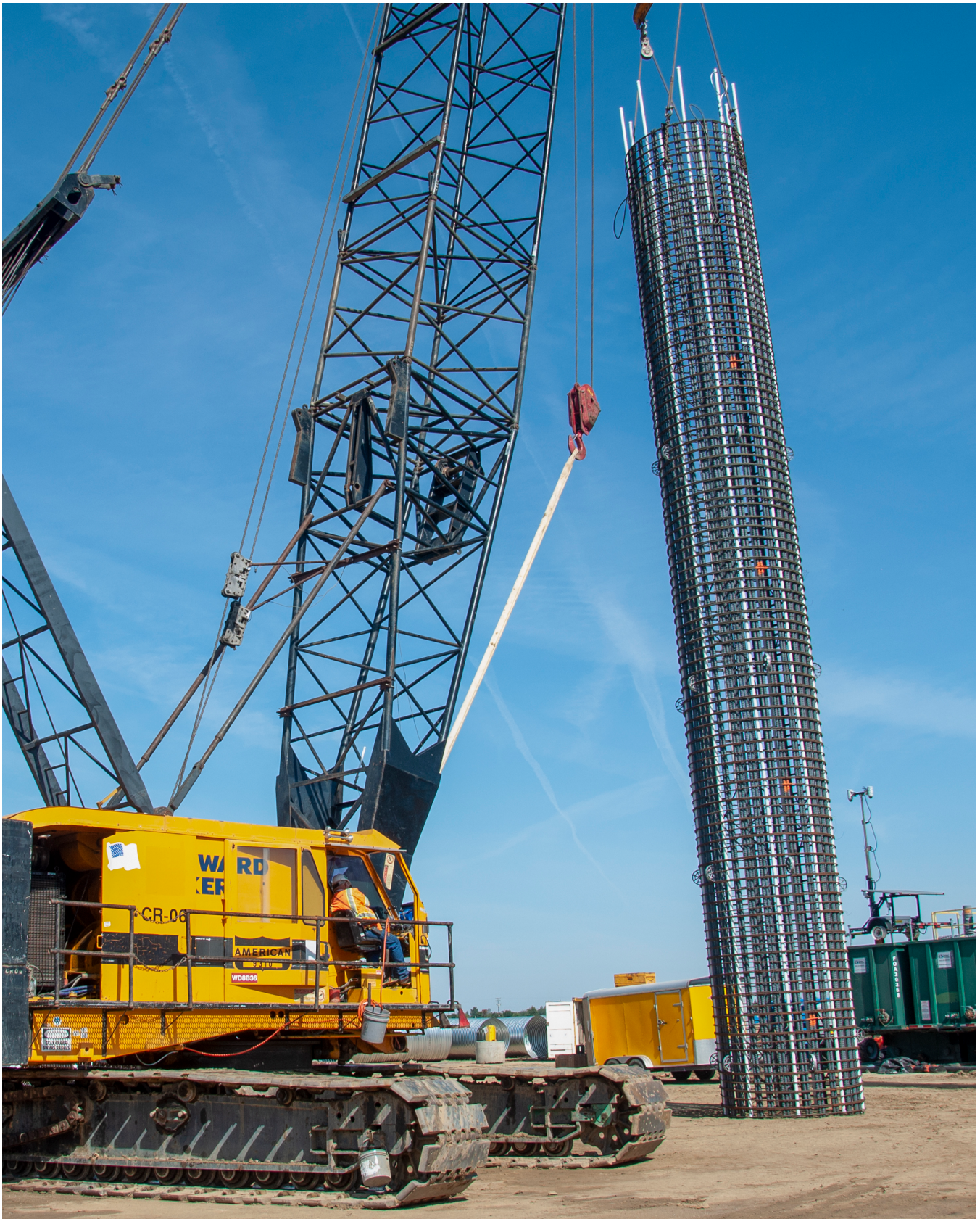
PHOTO: Rebar cages are one of the early stages in creating columns that will support a pergola.
